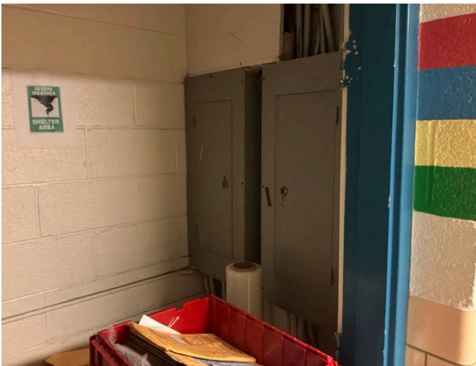
21 - ELECTRICAL DISTRIBUTION PANELS
